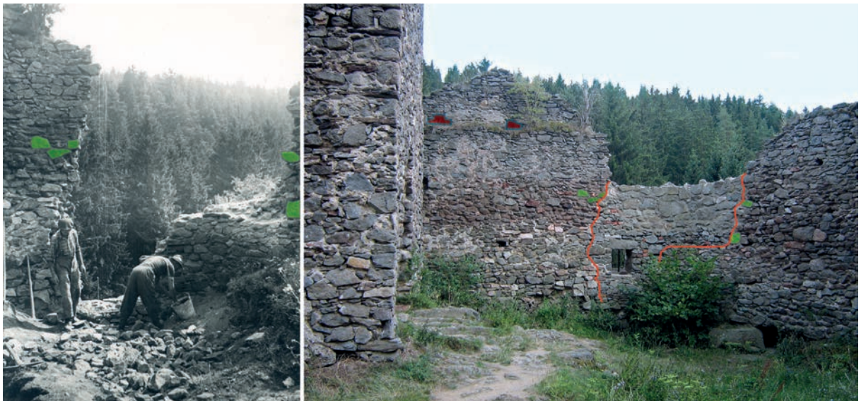
Fig. 7: The Mantelmauer of the Upper Castle. Left – original state of preservation in the 1960s. Right – contemporary situation after amateur preservation works.
